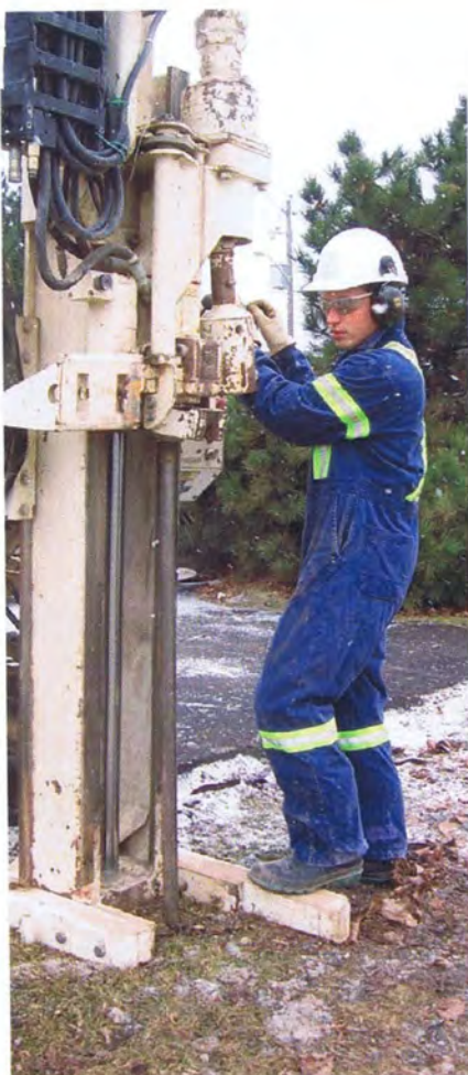
The assembled tool in preparation for driving by the direct push percussion drill unit.
